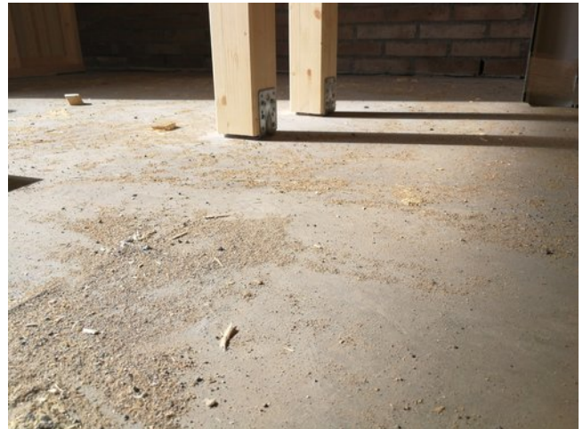
Rullakkovaraston runkotolpat irti betonista
